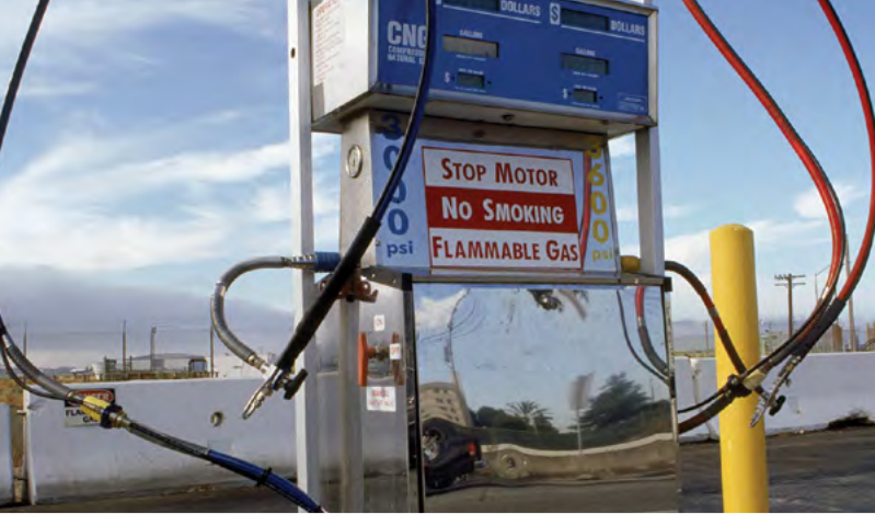
Compressed Natural Gas Dispensing
